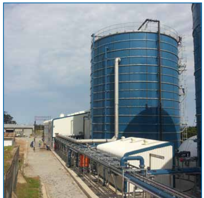
Bioreactor and filtration building.
