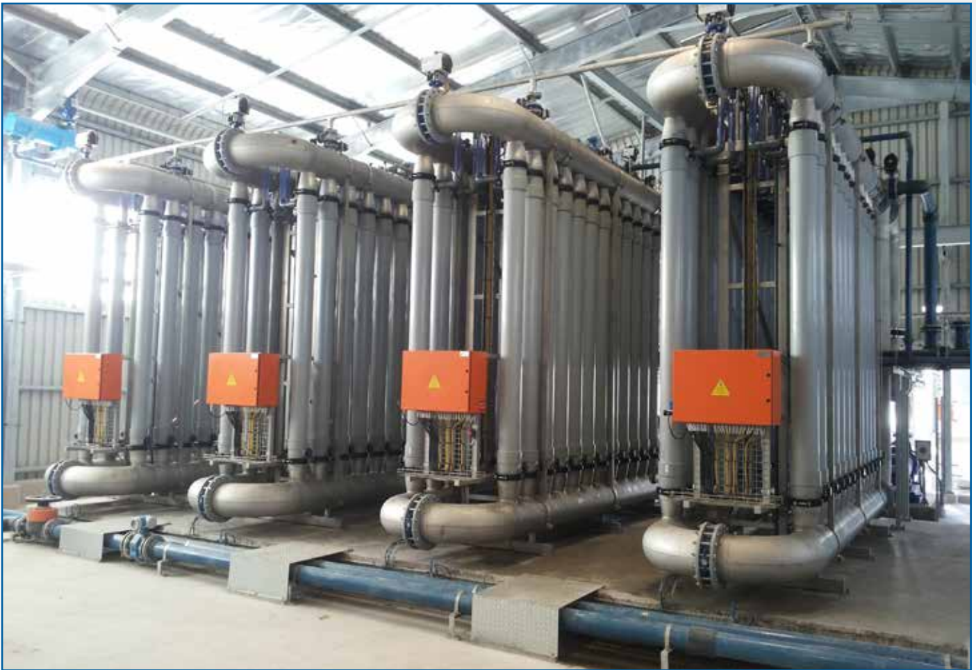
Installation of four Pentair® X-Flow™ Reverta Skids in collaboration with Veolia Biothane.
