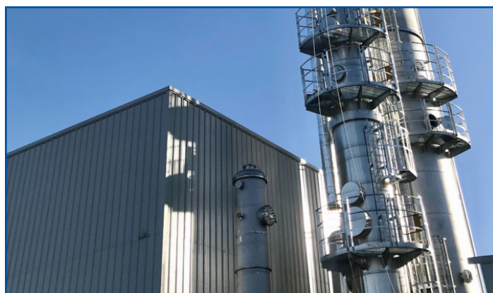
Scrubbing Tower at the TCE CCU plant in the UK. Image provided by Tata Chemicals Europe.
